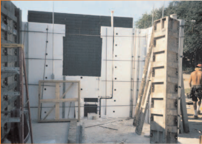
Western Forms donated the aluminum forming system, which utilized Dow Chemical Corporation's Thermomass technology foam system.
